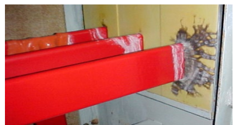
PD - damages insulation. Produce aggressive chemical by-products.
