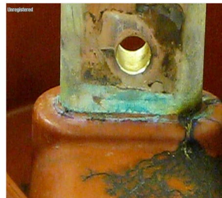
Partial discharge - Insulation
