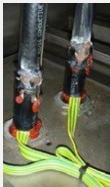
Partial Arcing in Single core terminations.
