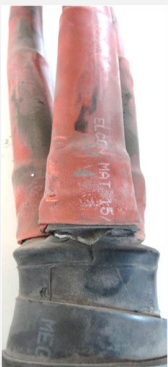
Partial Discharge in Tri core terminations.
